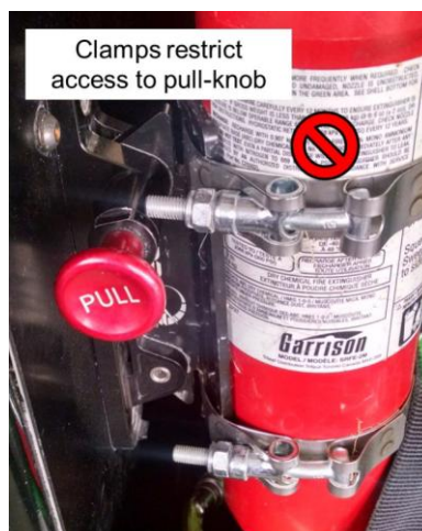
Figure B-51: Incorrect orientation of extinguisher clamps.
